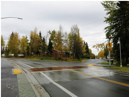
After: As part of a roadway improvement project, raised pedestrian crosswalks, widened shoulder striping and new pedestrian facilities and signage were incorporated to calm traffic. (photo courtesy of CRW Engineering Group)
