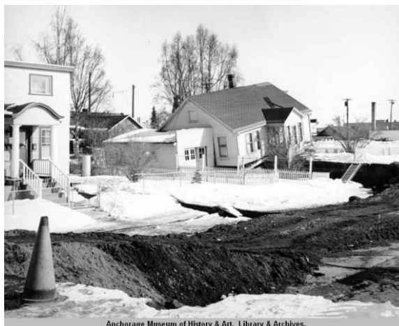
Figure 65. Earthquake damage at West 9 th Avenue and L Street, 1964. (Alaska Digital Archives, #AMRC-wws-4176-02)
