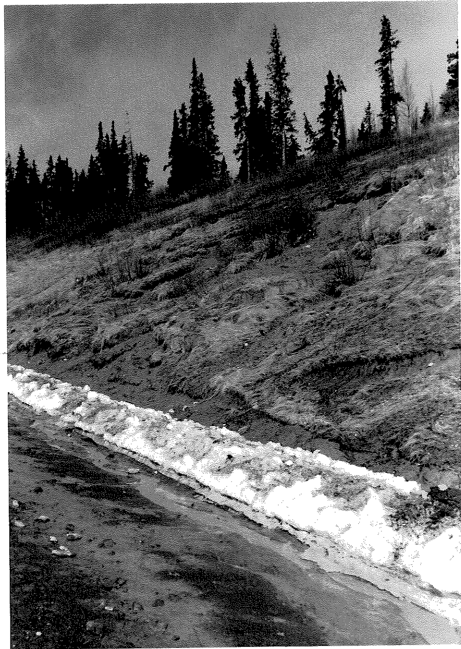
Figure 2a: Sediment from slopes where revegetation has failed to take hold or on slopes which have not been revegetated cause severe turbidity problems, particularly during "breakup."
