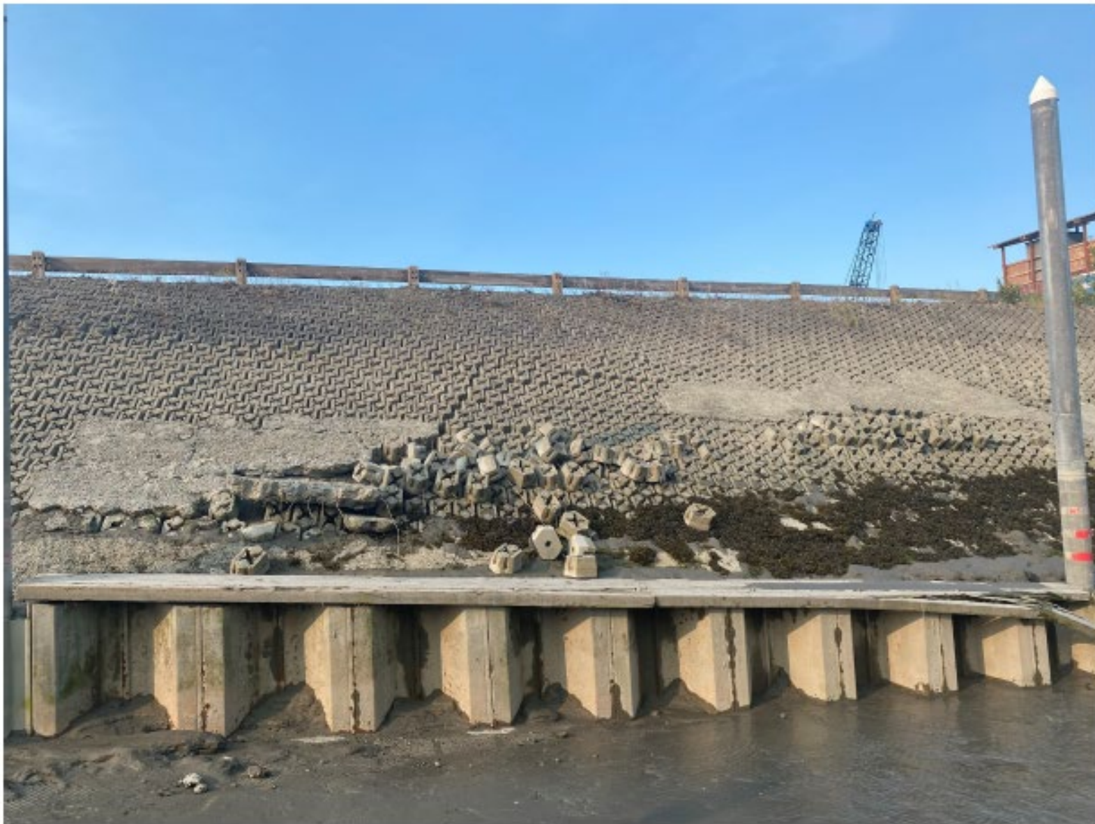
Photo 13: 2021 Project – South Backslope Failure (2021)
