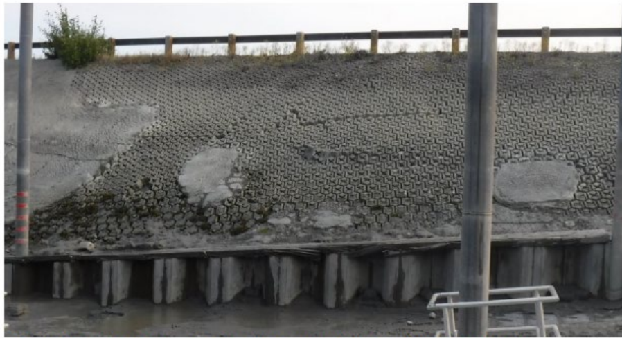
Photo 9: North Ramp – Break Line in Continuous ACB Mat (2021)
