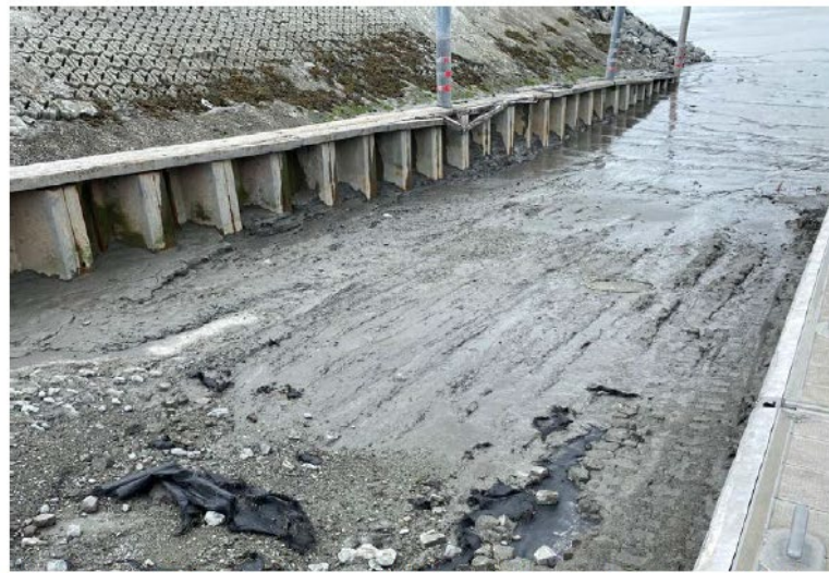
Photo 7: South Side ACB Ramp and Glulam Timber Fender Damage (2020)
