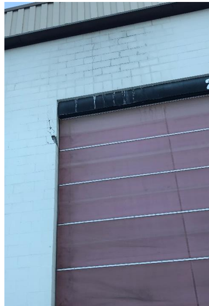
Photo 4: Mortar Failure Above Overhead Door #2
