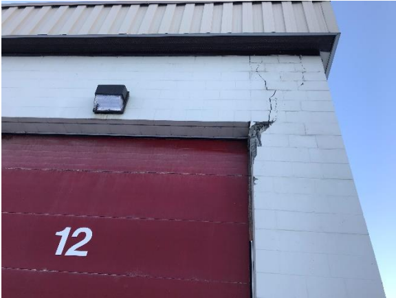
Photo 5: CMU Damage in Southwest Corner of Building
