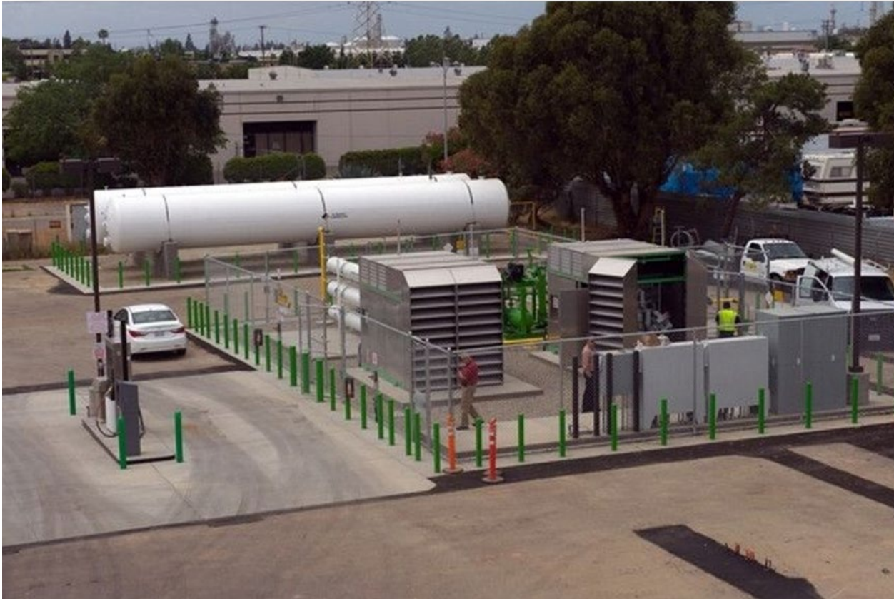
Figure 1-17: RNG Vehicle Fuel Production and Fueling Facility (Clean World Sacramento Biodigester)
