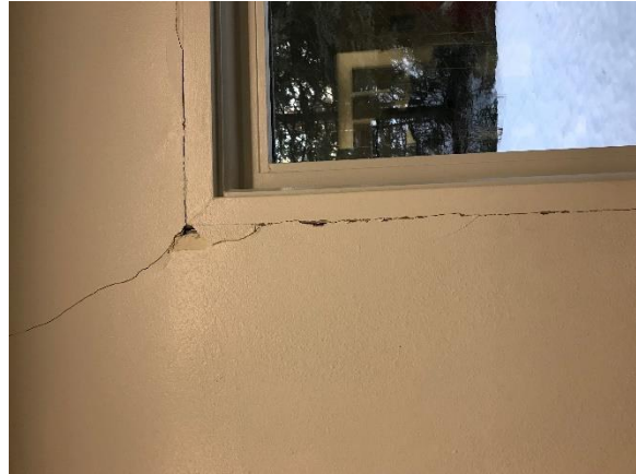
Photo 6: Typical Interior Drywall Damage
