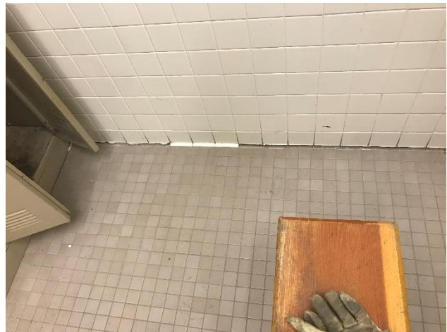
Photo 8: Typical Interior Wall Tile Damage
