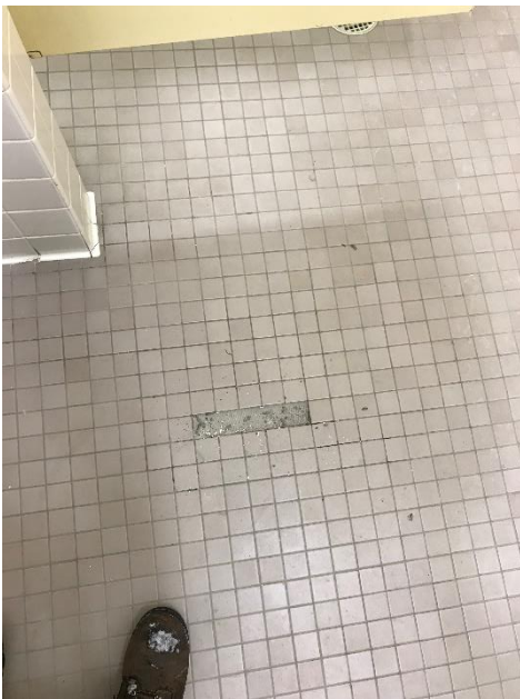
Photo 7: Typical Interior Floor Tile Damage
