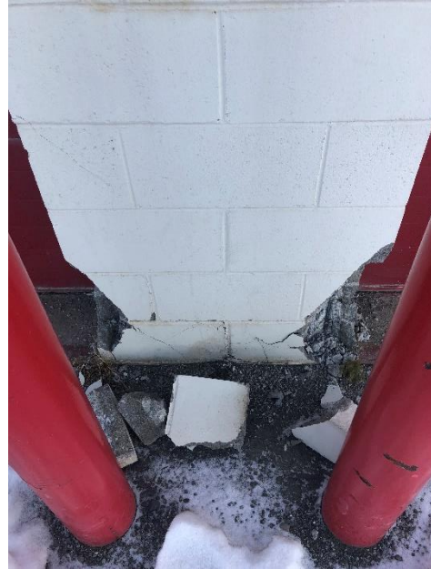
Photo 2: Typical CMU Blowout at CMU Columns
