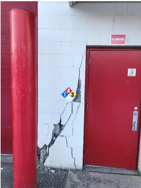
Photo 3: Significant CMU Block Damage to East Wall Near Administrative Area
