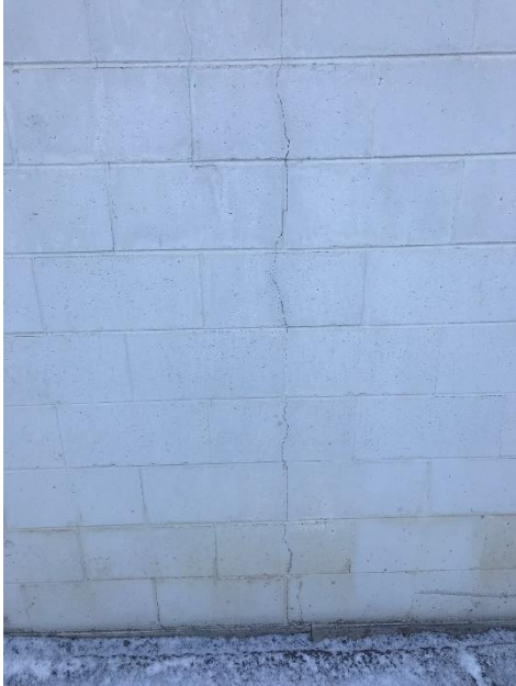
Photo 1: Typical Tight Cracking in CMU Blocks
