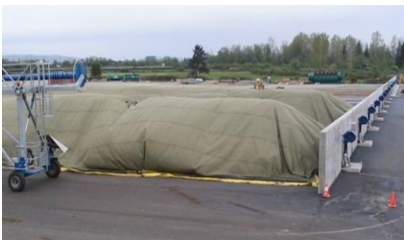
Figure 4.4-4: Membrane Covered Aerated Static Pile
